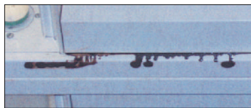
PCBs leaking out of metal casing.
