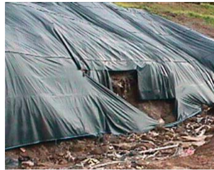
Storm drain failure
