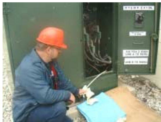
Figure 5. Transformer Sampling at Cooper
