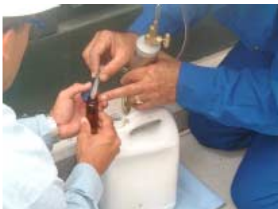
Figure 4. Transformer Sampling performed at SMHS and TI
