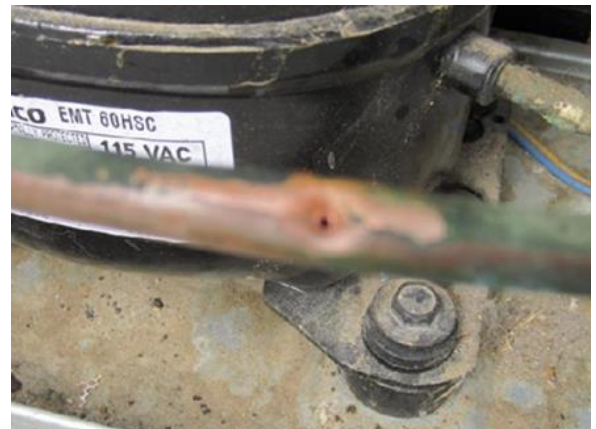
Figure 1: Drained Refrigerant lines will have a puncture mark.
