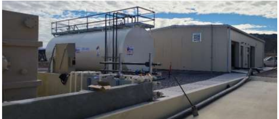
Photograph 1: Ethanol Storage Tank and Carbon Amendment Building
