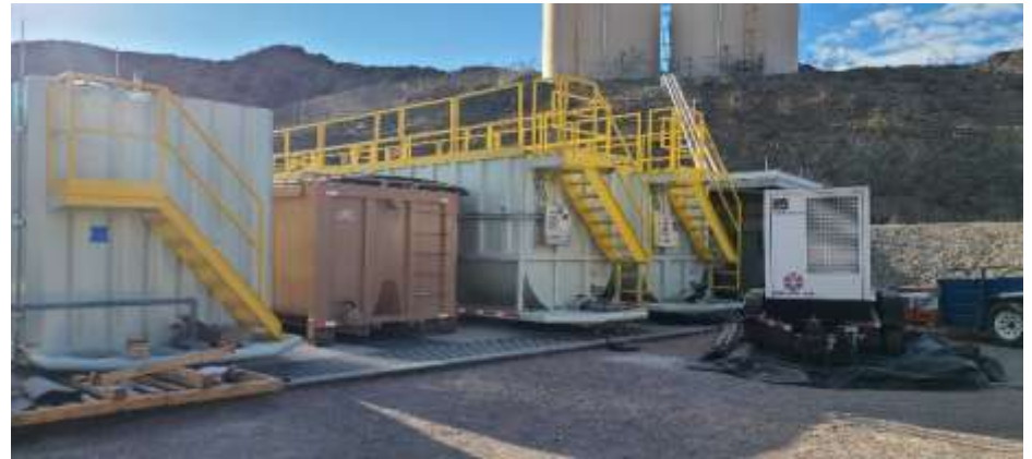
Photograph 2: Remedy Produced Water Conditioning System
