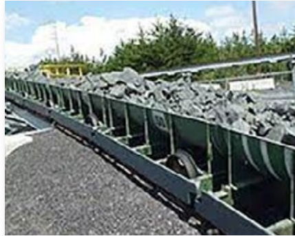
Cart conveyor (on grade)
