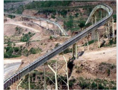
Pipe conveyor (on/above grade)
